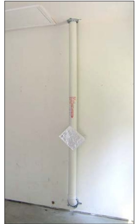
An example of a radon-control vent pipe.
